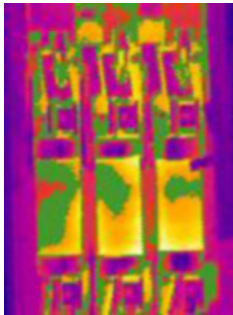
Figure 16.6 An isotherm in an infrared image of a fusebox
