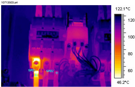
Figure 16.9 An infrared image of indoor electrical equipment (2)
