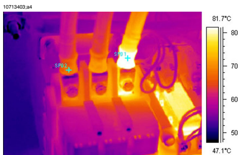
Figure 16.8 An infrared image of indoor electrical equipment (1)
